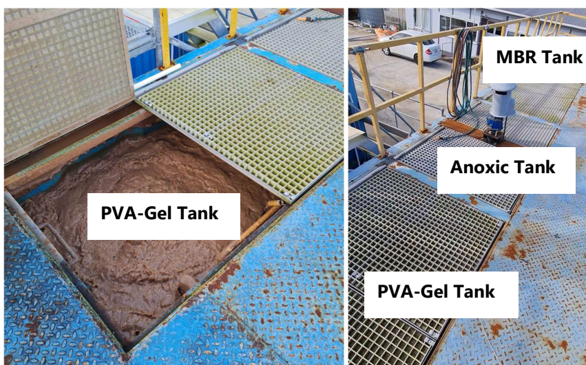
Figure 8: PVA-Gel and MBR Tanks
