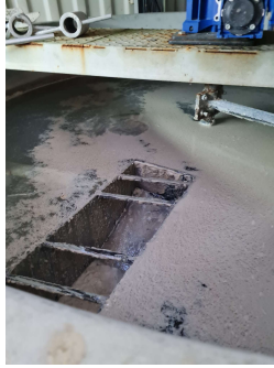
Figure 9: No thickened sludge on the DAF surface
