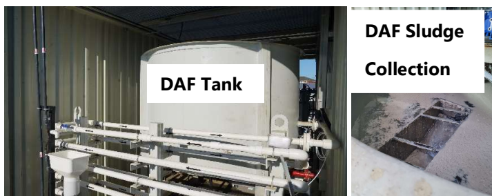
Figure 7: DAF Tank Side (Left) and Top (Right)
